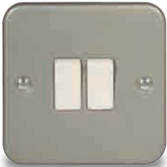
No visible plastic around switches
